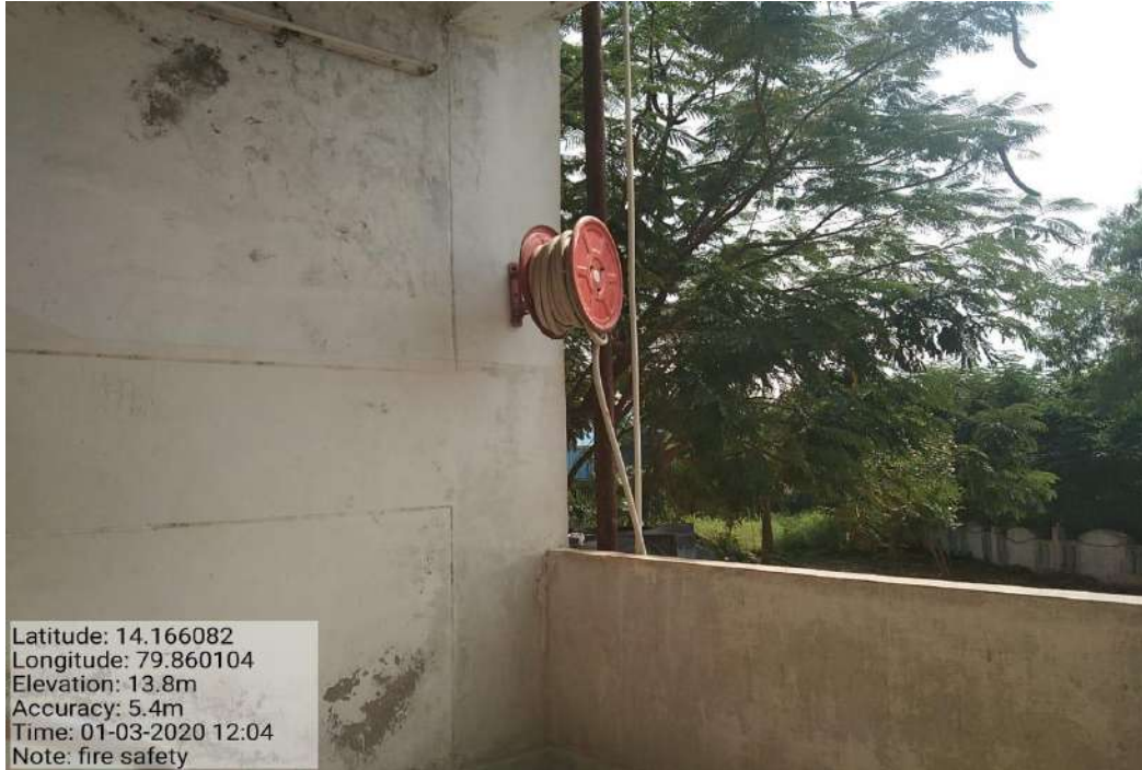
FIRE SAFETY on Floor
